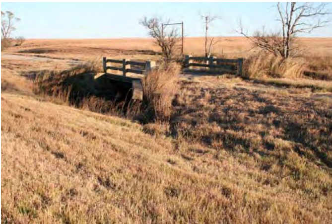
Caption: Restoration and rehabilitation of the historic U.S. 60 roadbed and bridges, that parallel much of the GSMB west of Pawhuska, as a bicycle/pedestrian trail could be funded under Transportation Enhancements categories numbers: 1, 2, 4, 6 and 7. Paul Daniel Marriott
