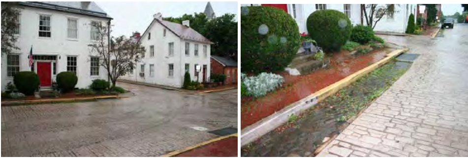
Caption: In Burkittsville, Maryland, CSS was utilized for an intersection improvement project by the Maryland State Highway Administration. Utility lines were undergrounded, historic stone gutters were redesigned and reconstructed to serve modern drainage needs, and the road was paved in concrete scored to reflect the pattern of the nineteenth-century stone pavement—the roughly-textured surface also serving as a traffic calming function. Photos: Paul Daniel Marriott
